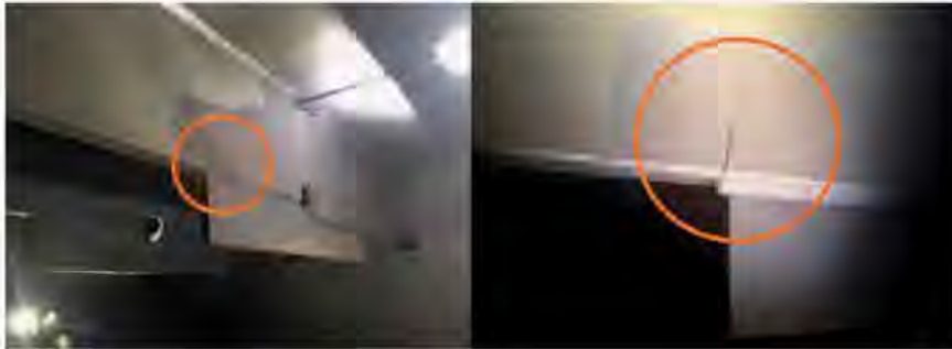
Fig. 3: Fatigue-induced cracks in the deck slab
