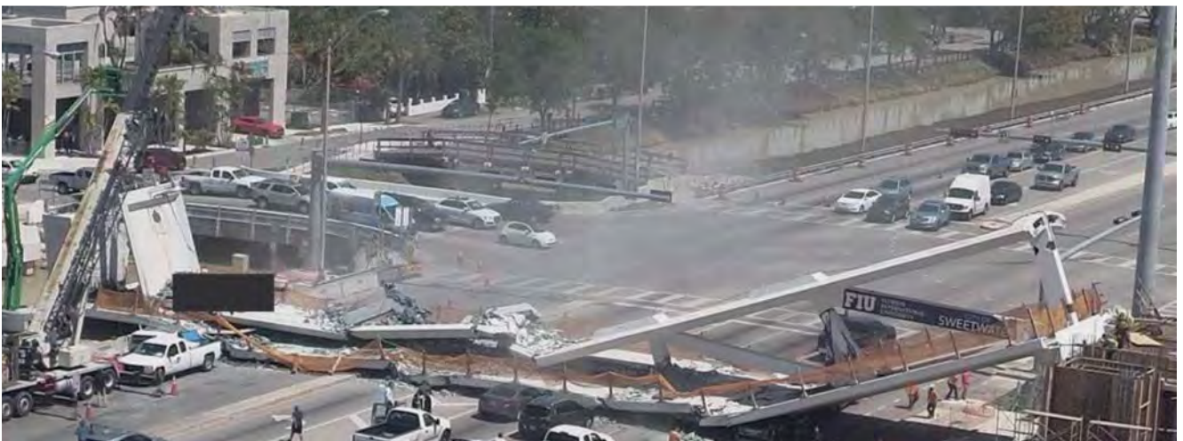
IN MARCH 2018, the pedestrian bridge spanning over SW 8th Street in Miami collapsed during erection due to node-point failure onto the heavily occupied road underneath.
